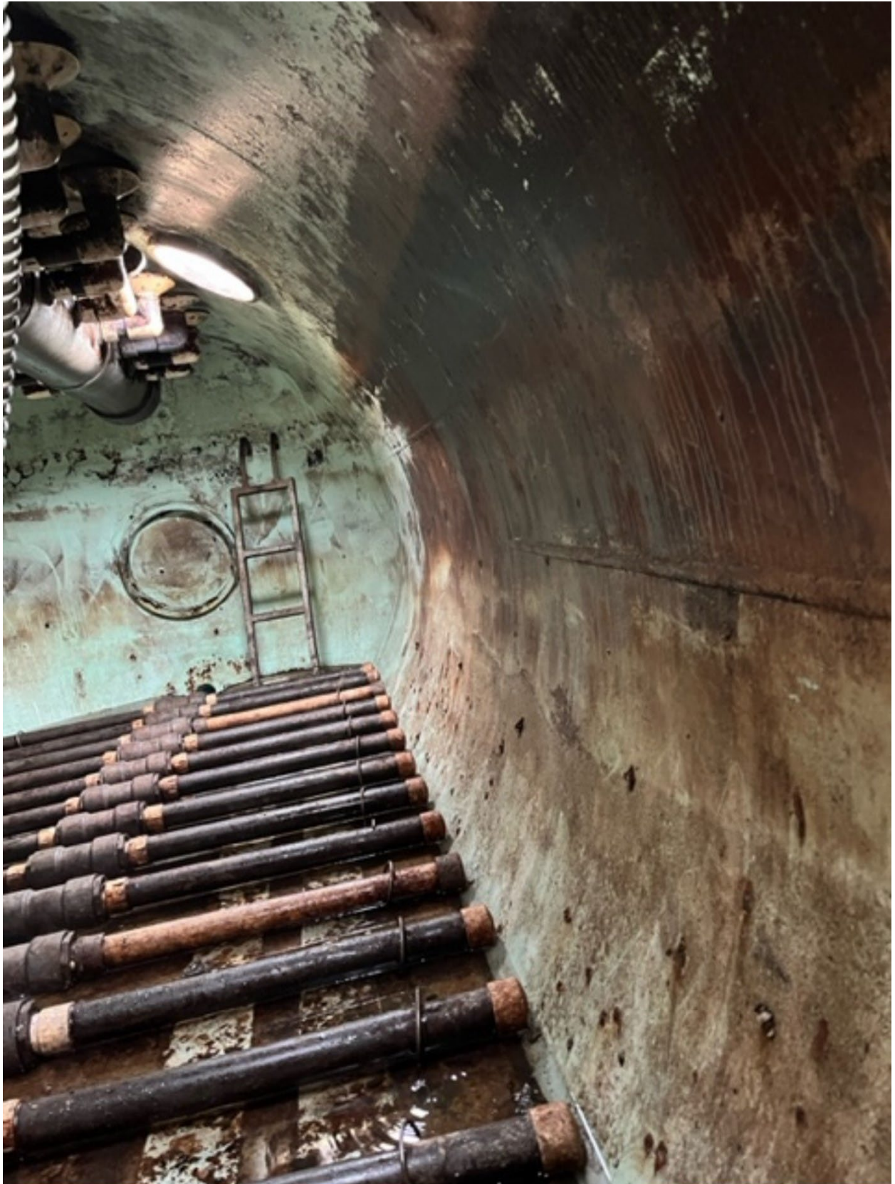
Attachment 1: Filter Tank Before
